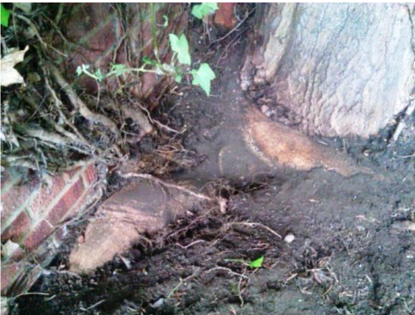
Fig. 10: Close-up showing root abutting the boundary wall and a girdling root passing northwards.
