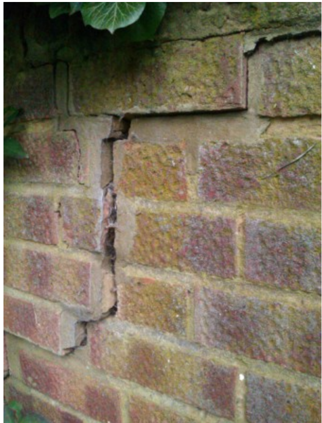
Fig. 2: Close-up of damage showing displacement by 12mm to the south west.
