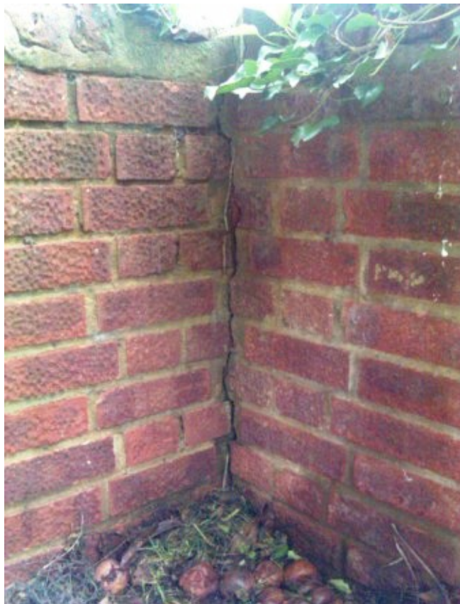
Fig. 4: Crack to north west of T1 where the damaged wall (left) meets the undamaged wall at the rear of xxx (right).
