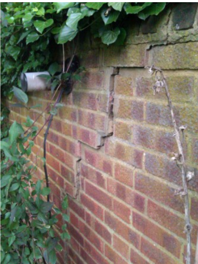
Fig. 3: Alternative view of damage.
