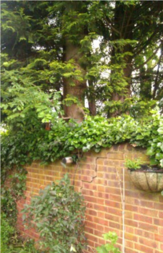
Fig. 1: General view of trees T1 & T2 and the damaged wall.
