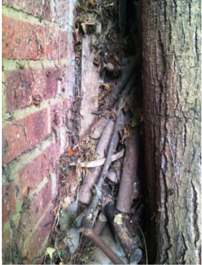
Fig. 6: Close-up after removal of hazel rods showing wood packed in between T1 and the wall.
